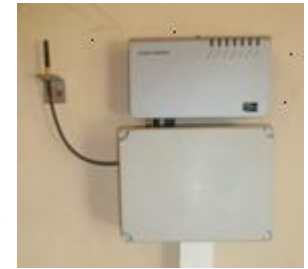
On-line monitoring system
