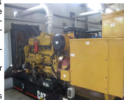
GEF projects substitutes expensive diesel generation on the island Brava
