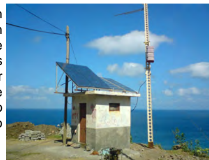
Telecommunication tower powered by PV in remote areas on the island São Nicolau
