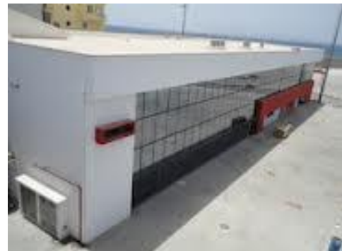
Figure 24: Passenger Maritime Station of Porto Novo, Santo Antão – south and west façade glassed. The installed AC units revealed inadequate during operation. AC Condensers placed in the searing heat of the roof.
