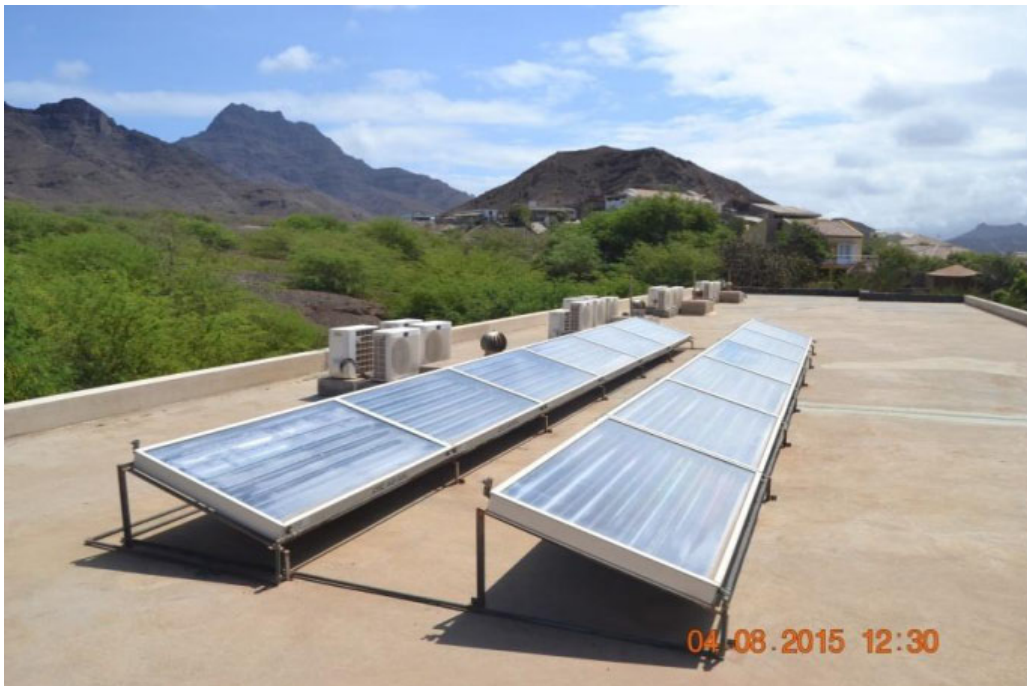
Figure 5: Circulated system, indirect type using CPC AO SOL Collector (FOYA BRANCA Hotel, in S. Vicente)
