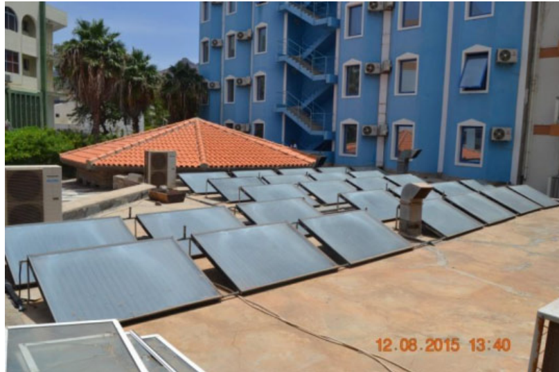
Figure 8: MINDEL Hotel flat plate solar collector (1.7 x 1.2 m) unbranded Italian made
