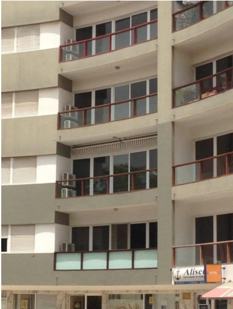
Figure 27: Condensers of compression type AC units in real estate investment in S. Vicente
