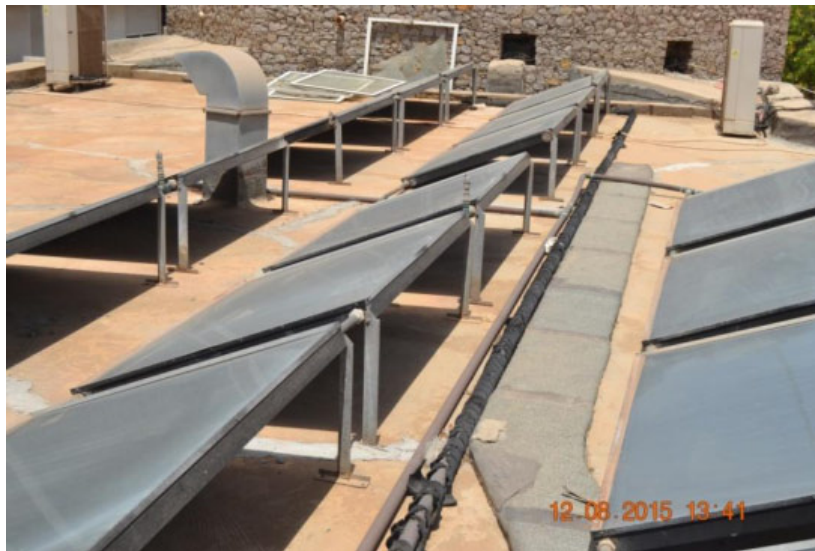
Figure 9: MINDEL Hotel, poorly insulated copper piping carrying hot water to storage tank
