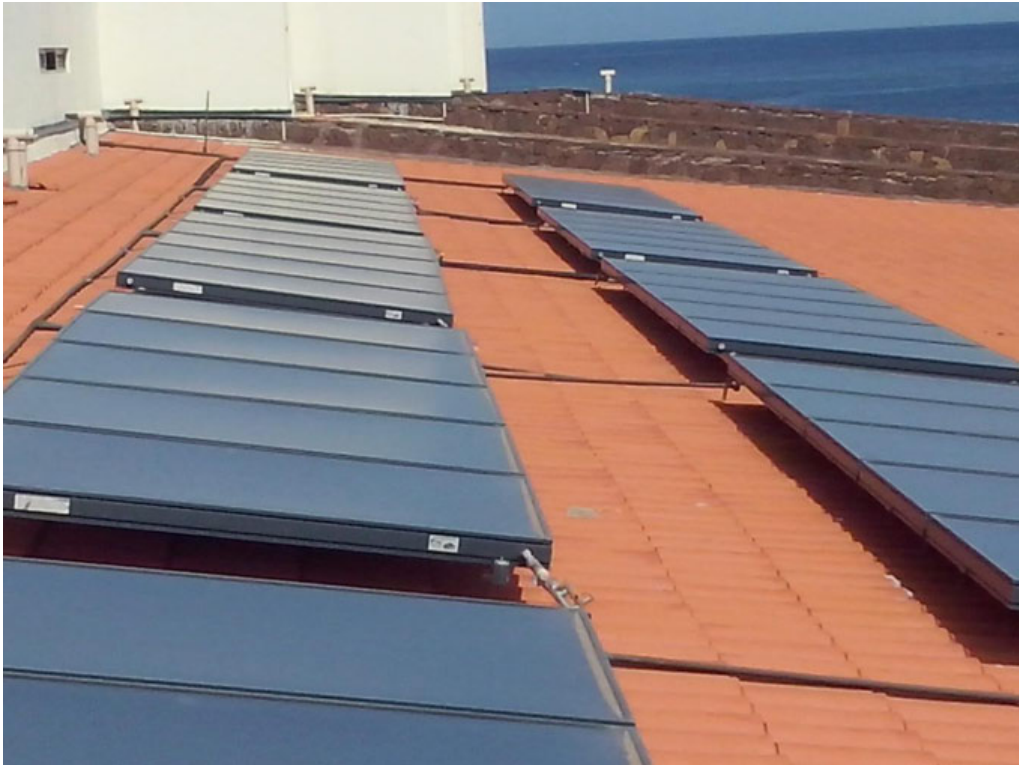
Figure 14: Two rows of solar collectors at PESTANA TROPICO Hotel
