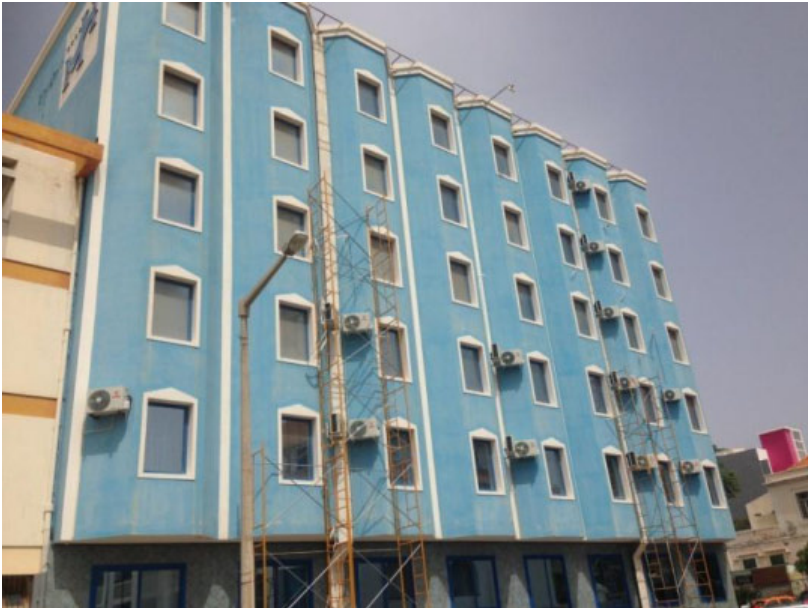
Figure 26: Condensers of compression type AC units being mounted in a hotel in S. Vicente (damaging the façade aesthetic)
